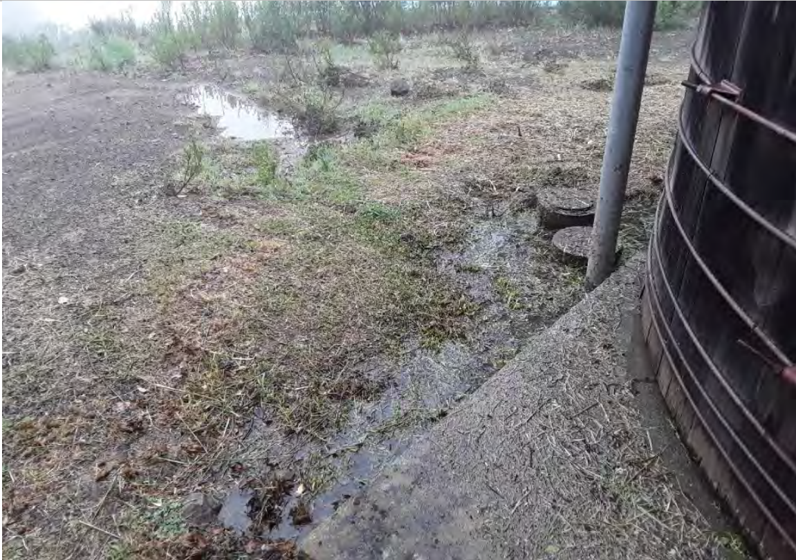
Photo 1: Wallan tank site looking south. Note upland conditions around the tank with pooled water from tank leak. This area was not considered wetland due to the completely artificial conditions and lack of hydrophytes and hydric soils. Photo taken April 19, 2022.
