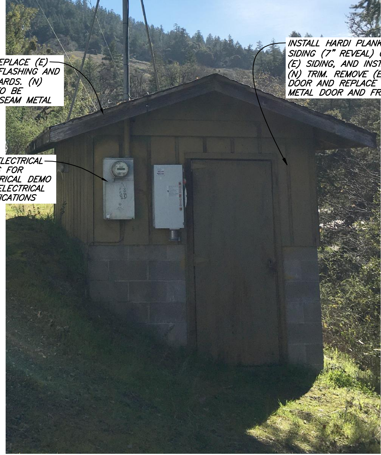
PUMP STATION EXTERIOR
