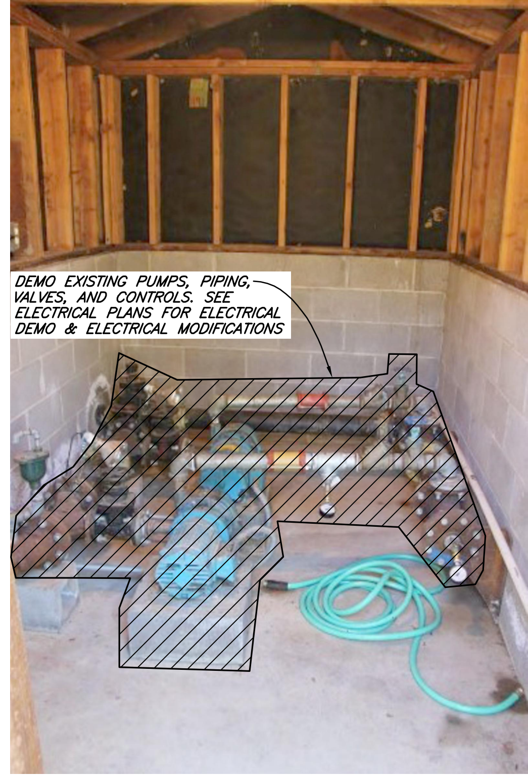
PUMP STATION INTERIOR
